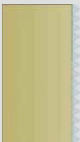
This leaves minute white/courless crystals at the surface (known as Efflorescence)
